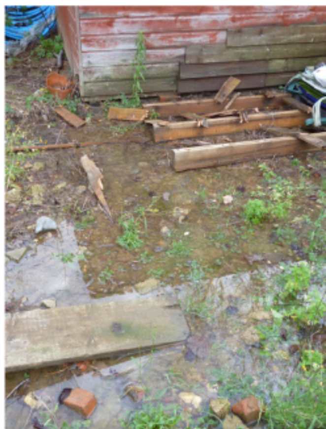
Flood - end of a Garden < 50 ft from Area 7a
