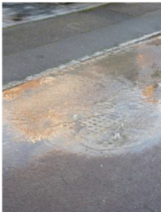
Hearne Drive Sewer Overflow
